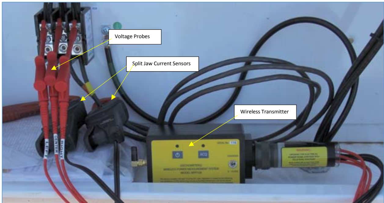
Figure 5 – Portable Wireless Power Probe Installed Temporarily inside Switch Box.
